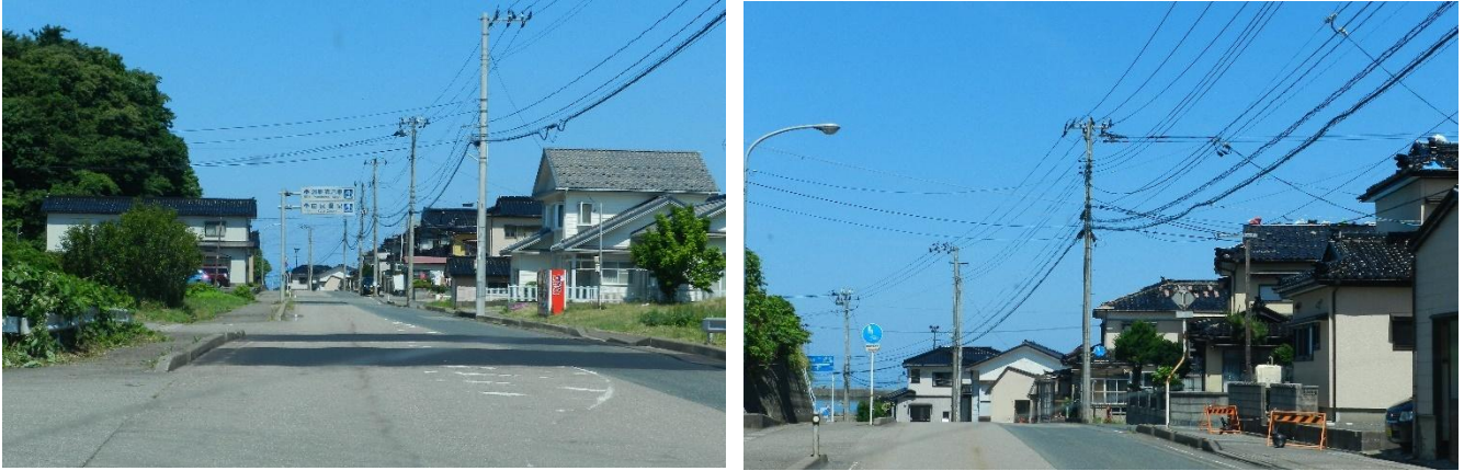
Fig. 3 Damage due to the earthquake rocked at June 18, 2019. The location is given in Fig. 1. a) Collapse and waving ("Jinami") of road (after restoration of the collapse) in Yura, Tsuruoka City, Yamagata Prefecture. Photo in June 26, 2019 (Left photograph). b) Damage of wooden house in Yura, Tsuruoka City, Yamagata Prefecture. Photo in June 26, 2019 (Right photograph).
