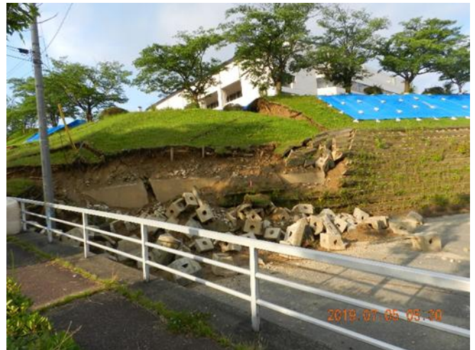
Fig. 8 Damage due to the earthquake rocked at June 18, 2019. Collapse of artificial slope on the side of the gymnasium ("Sanpoku Sougou Taiikukan") in Fuya, Murakami City, Niigata Prefecture (photo in July 5, 2019). The location is given in Fig. 1.
