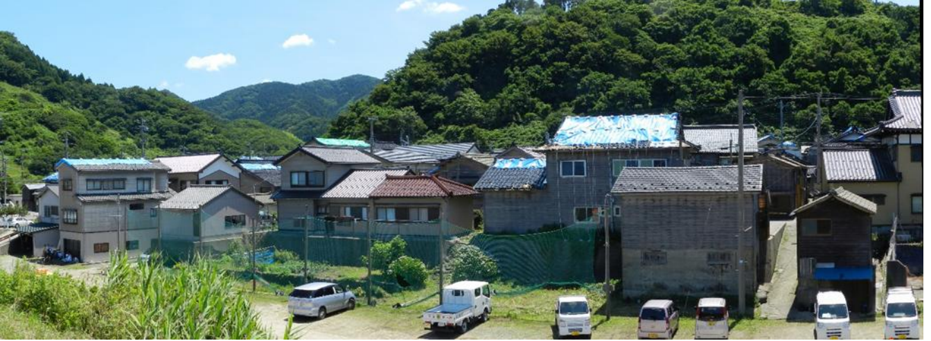
Fig. 4 Damage due to the earthquake rocked at June 18, 2019. The location is given in Fig. 1. Destruction of tiled roofs of wooden houses and their emergency restoration using "Blue sheets" in Koiwagawa, Tsuruoka City, Yamagata Prefecture. Panoramic photograph taken in June 26, 2019.
