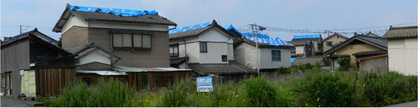
Fig. 6 Damage due to the earthquake rocked at June 18, 2019. The location is given in Fig. 5. Destruction of tiled roofs of wooden houses and their emergency restoration using "Blue sheets" in Nezugaseki (near JR Nezugaseki Station), Tsuruoka City, Yamagata Prefecture. Panoramic photograph taken in July 5, 2019.
