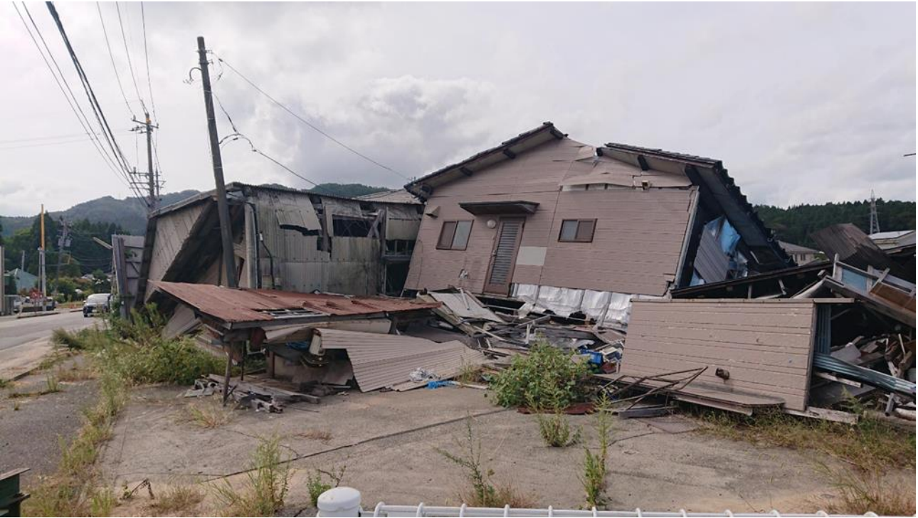
Fig. 8 The collapsed house in Yokoji-machi, Wajima City (Fig.1-a-⑦).
