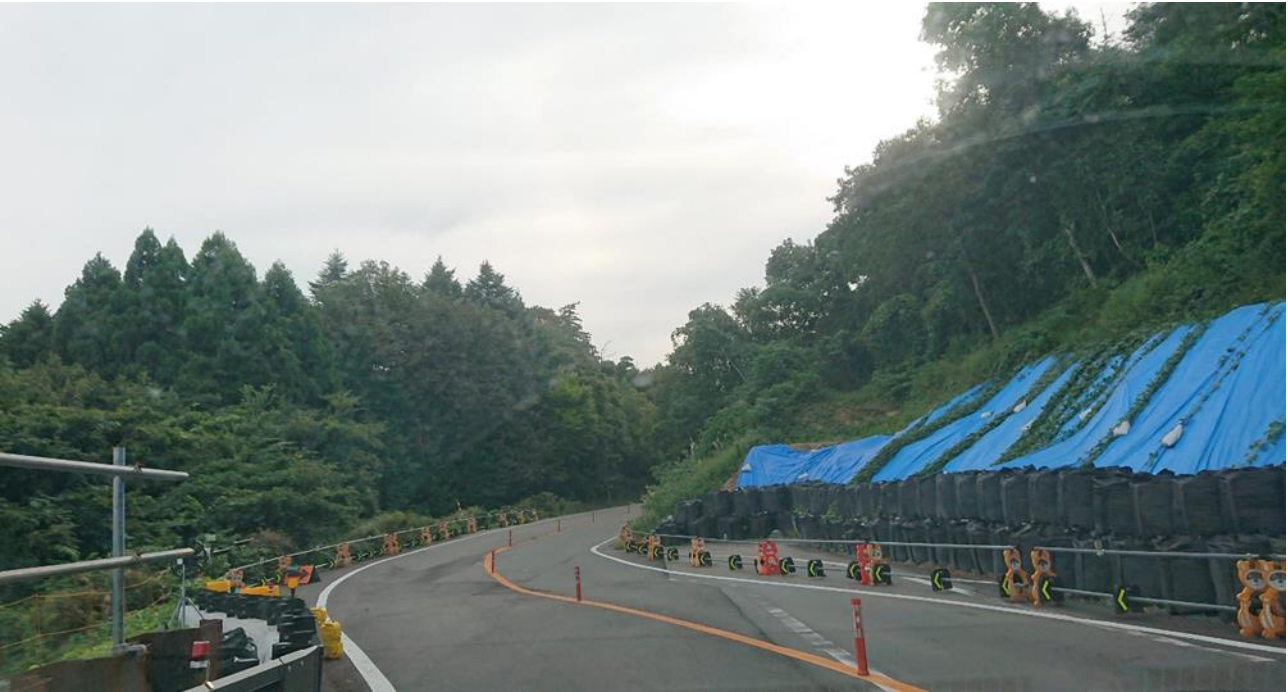
Fig.2 Earthquake restoration work is underway along Noto Satoyama Kaido. Located in Nakajima-machi, Nanao City, Ishikawa Prefecture (Fig.1-A-①).
