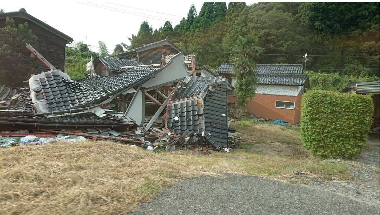
Fig.3 11 months after the disaster, many collapsed and uninhabitable houses can be seen. Located in Kawashima, Anamizu Town, Housu District, Ishikawa Prefecture (Fig.1-A-②).
