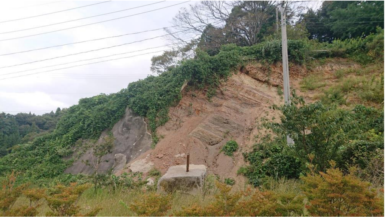
Fig. 5 A mountain slope collapsed due to an earthquake along Prefectural Route 1 in Miimachi-hongo, Wajima City (Fig.1-a-④).
